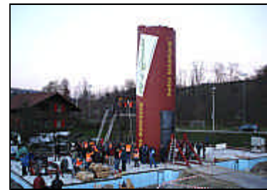
The massive storage tank was installed just after construction began two years ago (Jenni)
